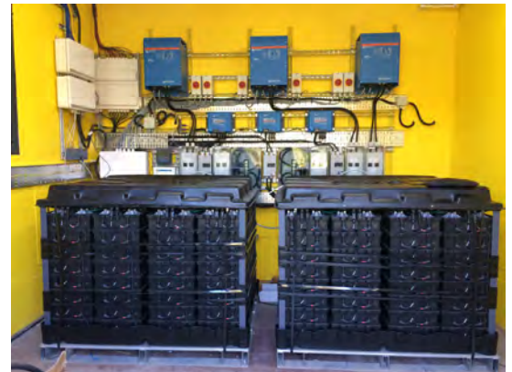
Figure 32: The Aquion batteries inverters and charge controllers
