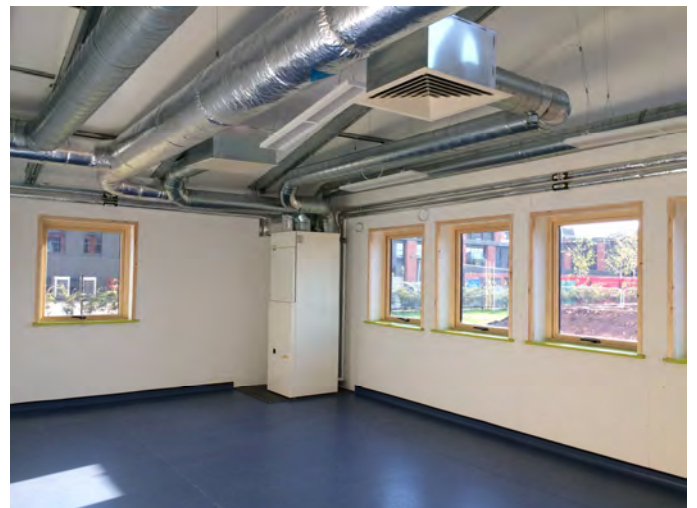
Figure 26: The Genvex unit and air distribution ductwork
