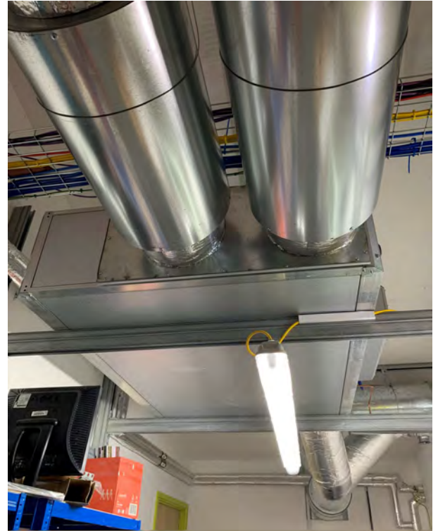
Figure 27: MVHR unit and duct entry point from TSC
