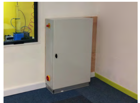
Figure 24: The control box #1
