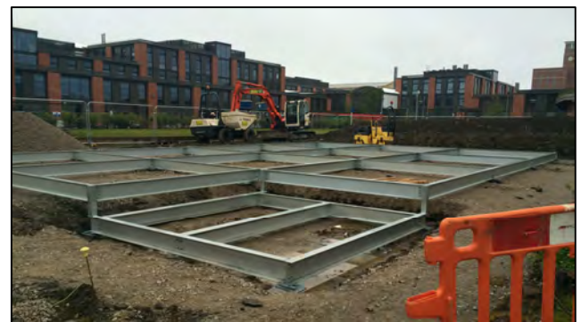
Figure 17: The steel screw pile foundations and the steel grid to support the building. The lower square in the foreground is the plant room, which is lower to enable flat access from the existing pavement.
