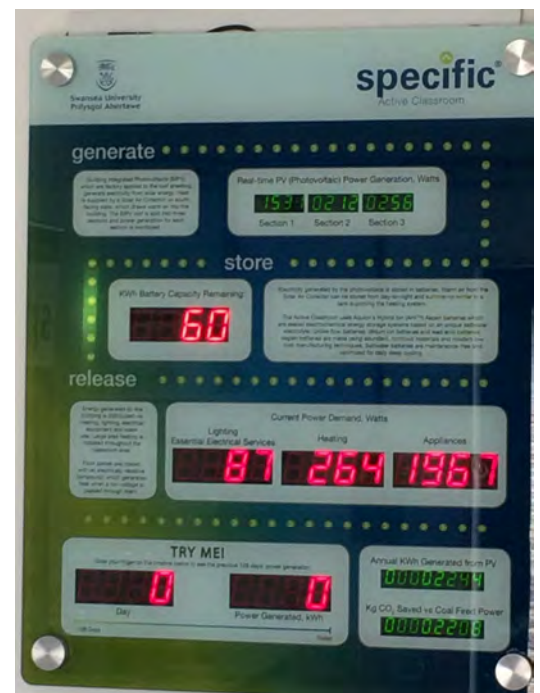
Figure 37: Display screen linked to the monitoring system
