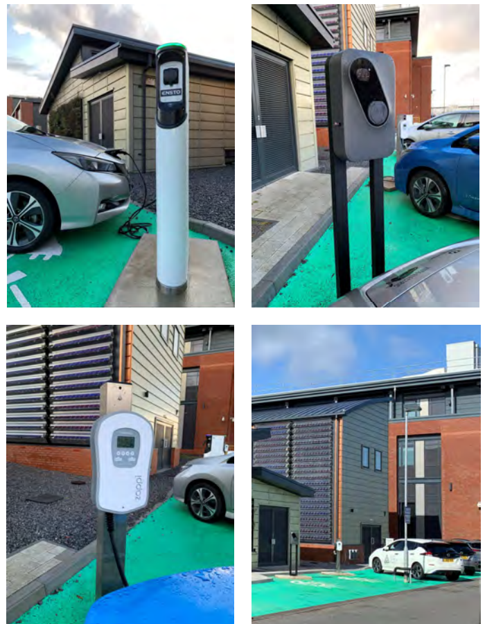
Figure 72: Smart EV chargers outside the Active Buildings
