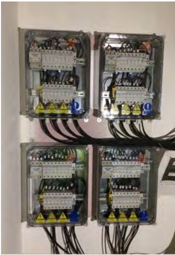
Figure 49: PV connection panel
