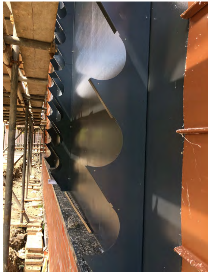
Figure 60: Brackets for PVT system
