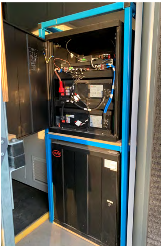
Figure 24: The battery system
