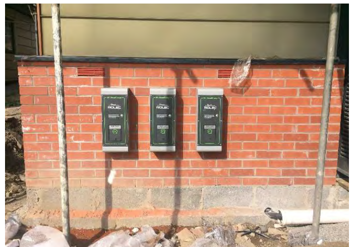
Figure 58: Wall mounted Electric vehicle charge points
