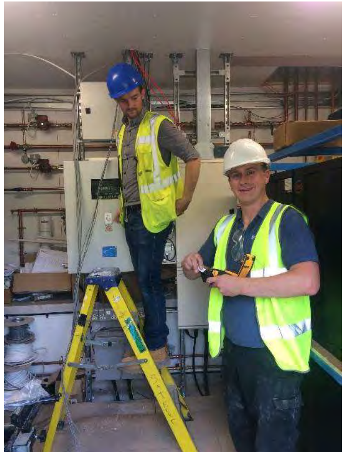
Figure 65: Smart Systems Engineers, Dr Richard Lewis and Tom Griffiths in the Plant Room
